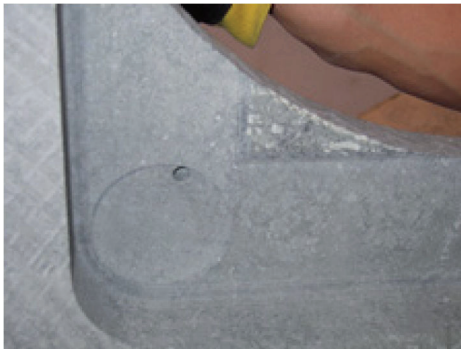
28. These two milled holes fit over the bracket just installed, holding the top panel in place.
